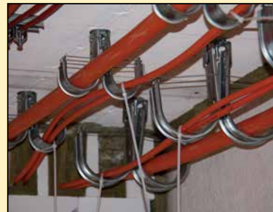
J-Hooks and cables in fire chamber before fire test
