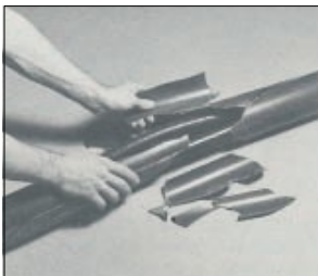
Remove damaged or faulty ducting
